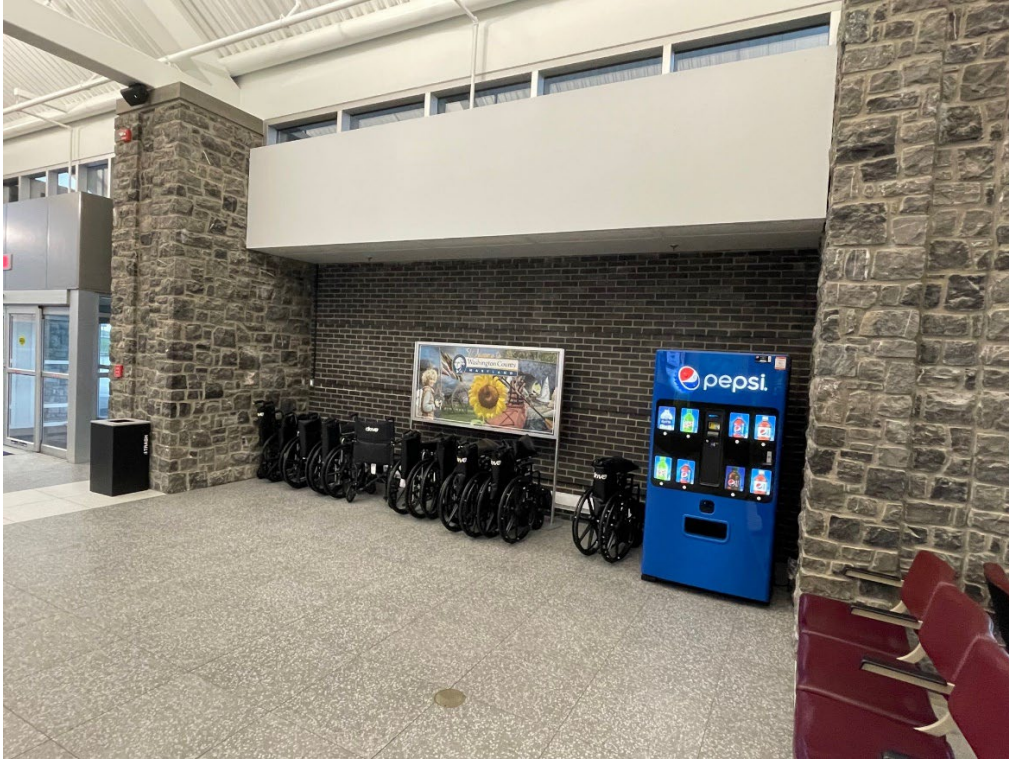
Figure 2. Concession Option “1” Space 108 (Terminal East Wing). Approx. 20.5’ W x 12’ D (246 SF TOTAL) incl. 20.5’ W x 5’ D (102.5 SF) for standing room/branded carpet(s) in front of counter (above)
