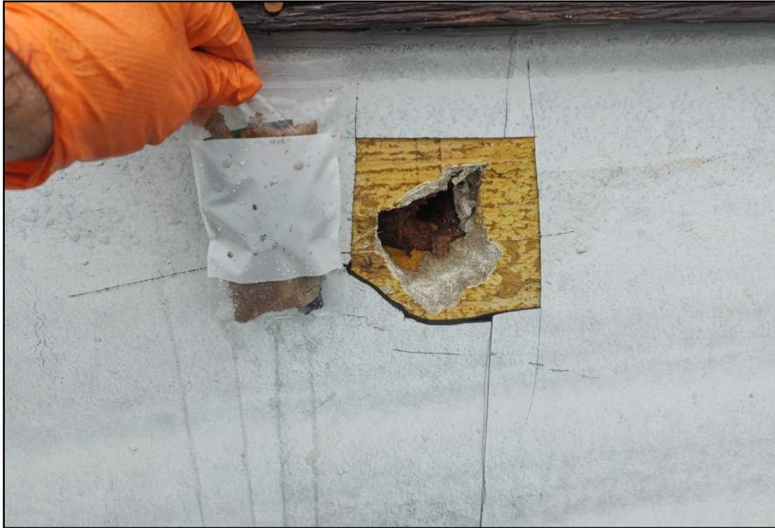
13. View of HA #20—Membrane, Rigid Fiber Board, and Cellulose-like Board located at the ~4-foot Wall at Roof Elevation Change between Western Low Main Roof and Upper Main Roof. Laboratory analysis reports a layer of this material contains 20% Chrysotile. Other layers examined by the laboratory were reported to contain Trace <1% Chrysotile, but such concentrations may be from contamination from the “Transite” layer.
