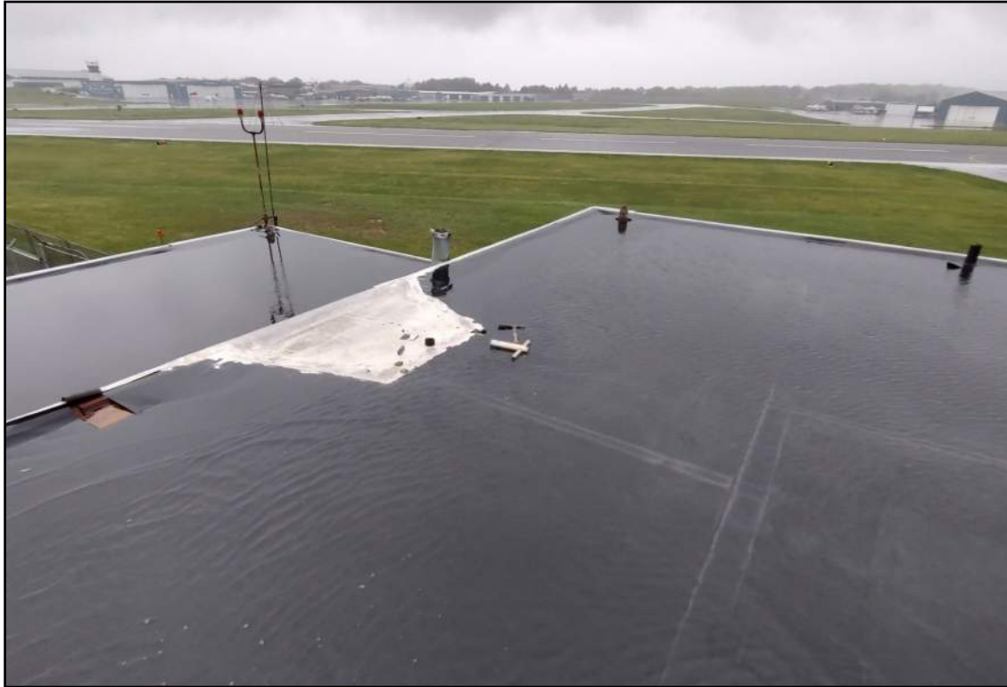
9. View of a portion of the Roof which was historically patched.
