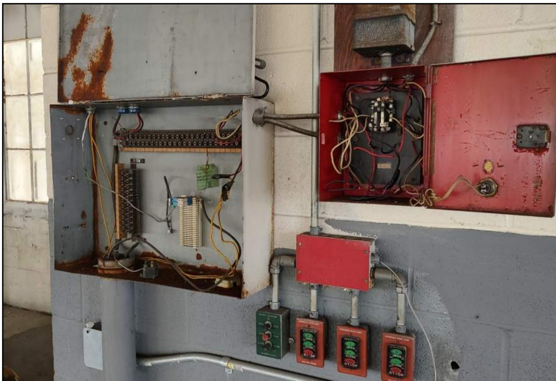
6. View of electrical panels within the Fire Station.
