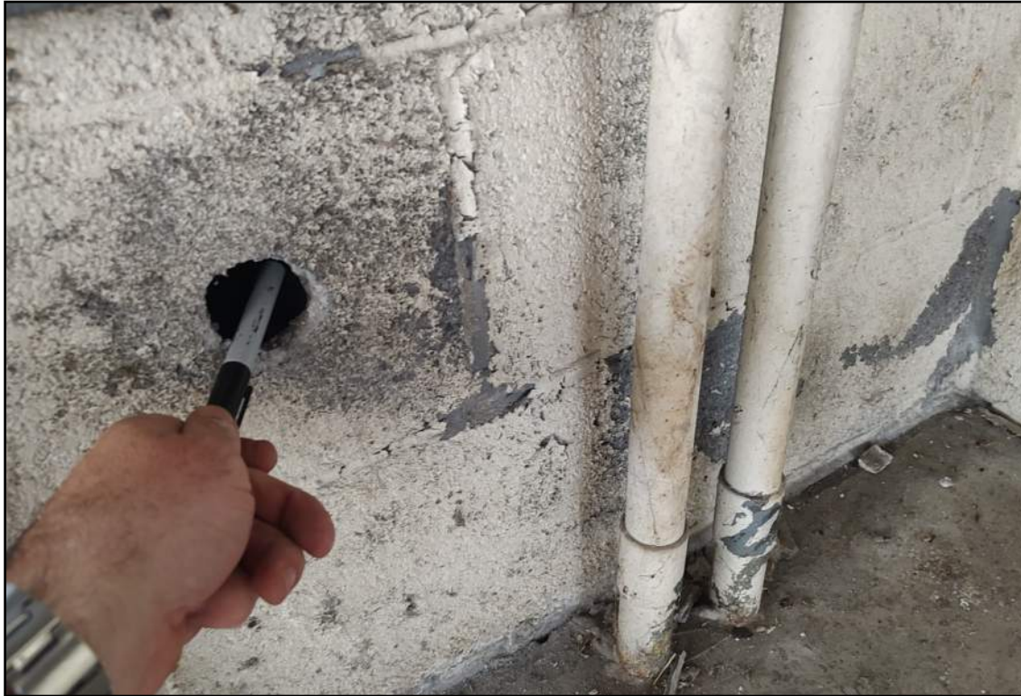
5. View of a test cut to inspect for the presence of Vermiculite within the CMU Block. Vermiculite was not identified in test cuts made by F&R.
