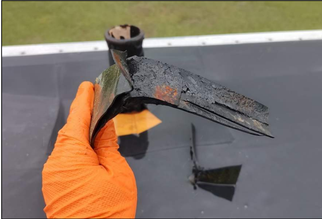
11. View of HA #18—Black Adhesive at Vent Pipe Penetration on the Upper Main Roof at the North Center Area at the Vent Pipe. Laboratory analysis reports this material contains 2% Chrysotile.
