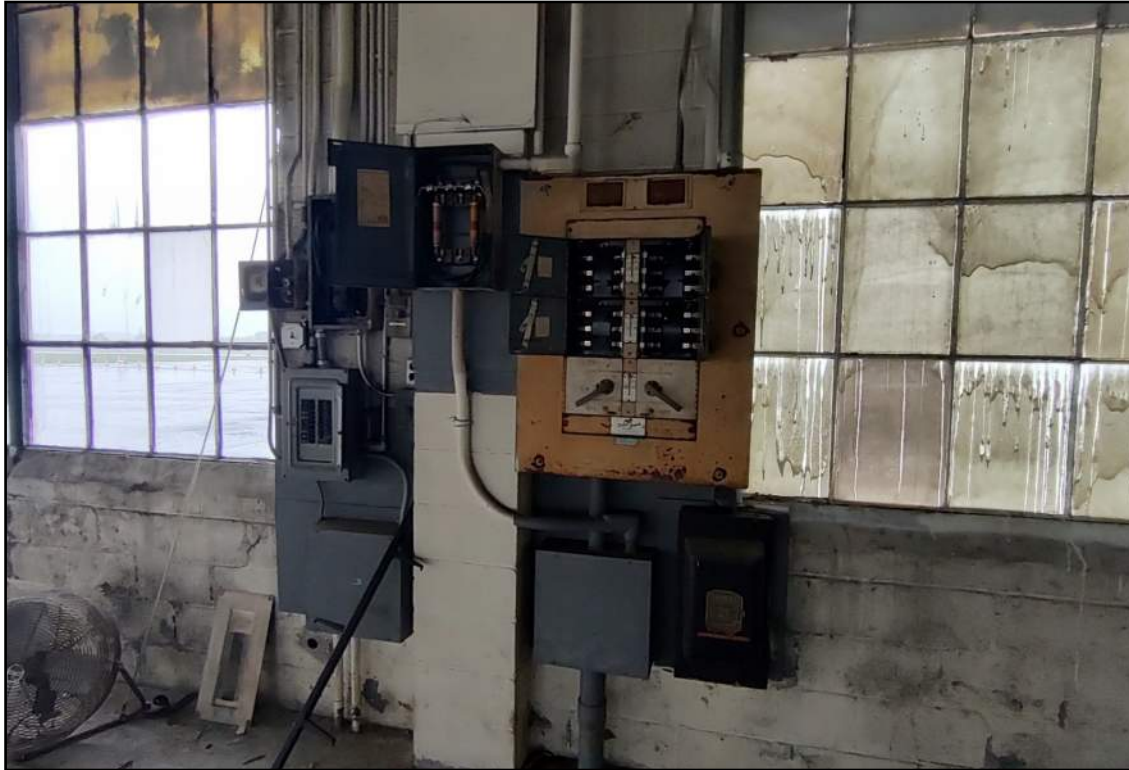
7. View of electrical panels within the Fire Station.
