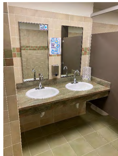
Women's Toilet Room Sinks
