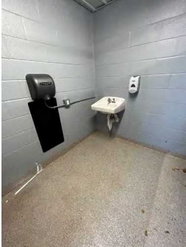
Women's Toilet Room Sink
