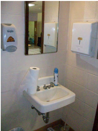
Women's Toilet Room Sink
