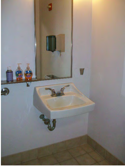
Women's Toilet Room Sink
