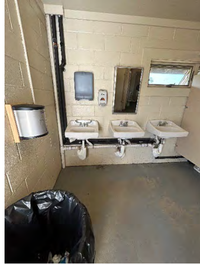
Women's Toilet Room Sinks
