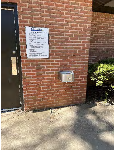
Drinking Fountain (Not in Operation)
