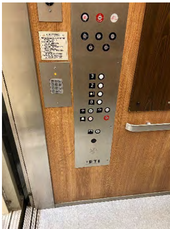
Elevator Control Panel
