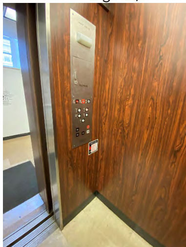
Elevator Control Panel
