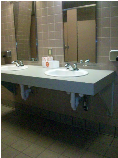
Women's Toilet Room Sinks
