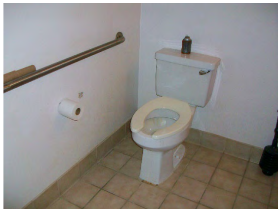
Men's Toilet Room Water Closet
