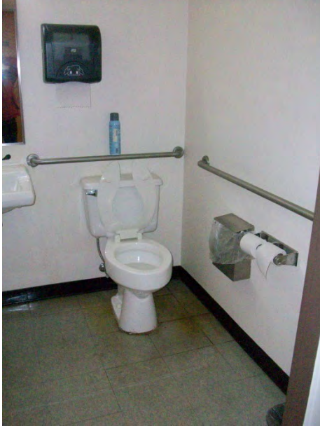
Toilet Room Water Closet
