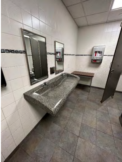
2 nd Floor Women's Toilet Room Sink
