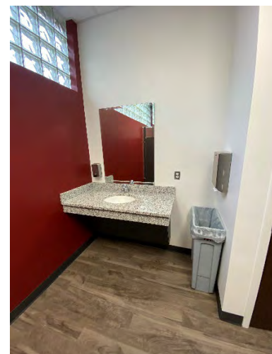
Women's Toilet Room Sink
