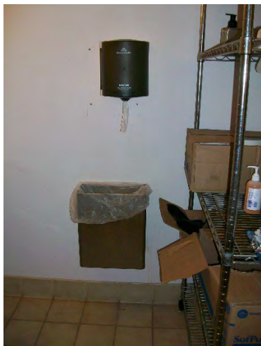
Men's Toilet Room Hand Dryer
