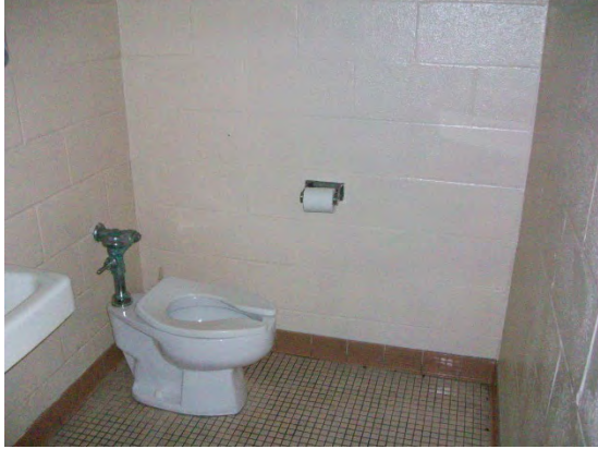
Men's Toilet Room Water Closet
