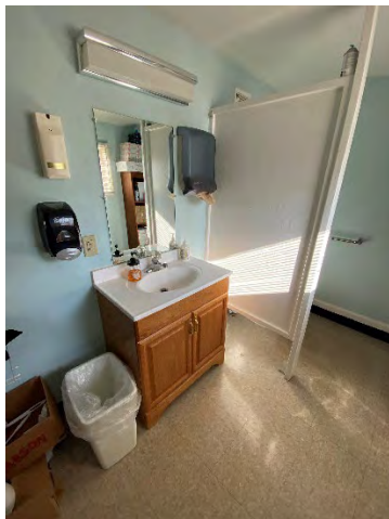
Women's Toilet Room Sink
