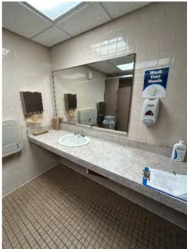
2 nd Floor Women's Toilet Room Sink
