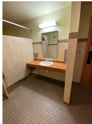
Women's Toilet Room Sink
