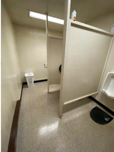
Men's Toilet Room Stall Fixtures
