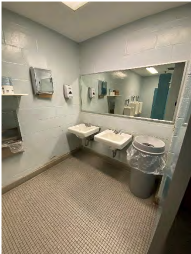
3 rd Floor Men's Toilet Room Sinks
