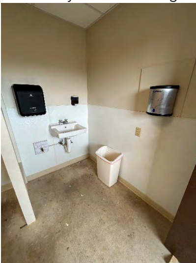
Men's Toilet Room Sink
