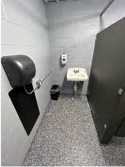
Women's Toilet Room Sink
