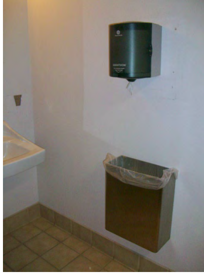
Women's Toilet Room Hand Dryer
