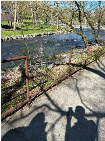
Broken Portion of Handrail on Pathway on Eastern Side of Bridge
