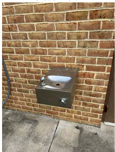
Drinking Fountain (Not in Operation)
