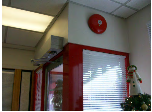
Main Entrance Door Closing Hardware & Fire Alarm
