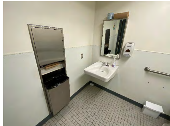
Women's Toilet Room Sink
