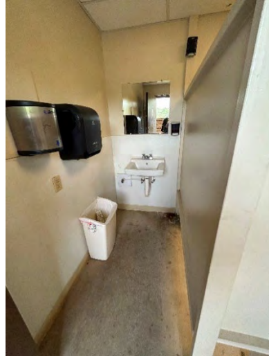
Women's Toilet Room Sink
