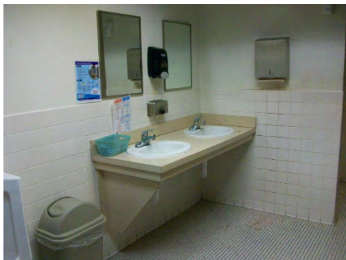
(Right) Men's Toilet Room Sinks
