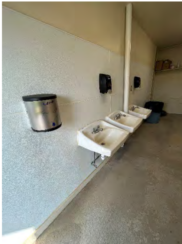
Women's Toilet Room Sinks
