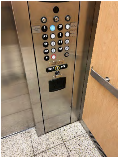
Elevator Control Panel
