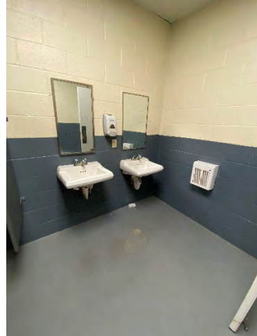
Multi-Purpose Building Men's Toilet Room Sinks
