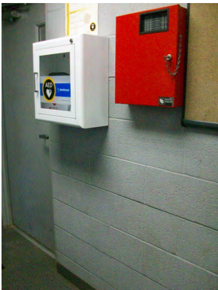
AED / Security Control Panel
