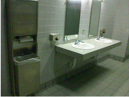
Men's Toilet Room Sinks
