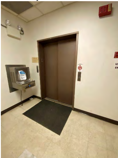
Rear Building Elevator & Drinking Fountain (Neither in Operation)
