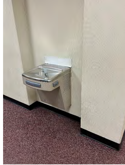
3 rd Floor Drinking Fountain
