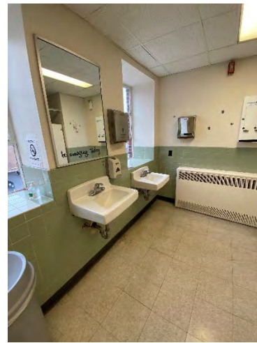
3rd Floor Women's Toilet Room Sinks
