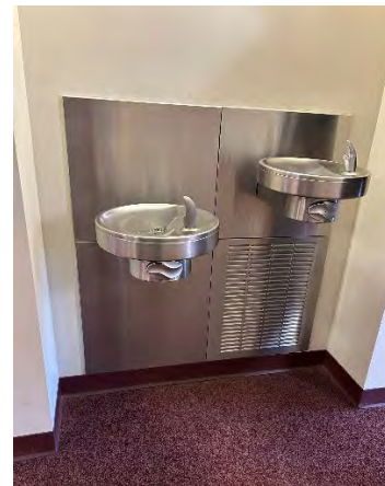
2 nd Floor Drinking Fountain
