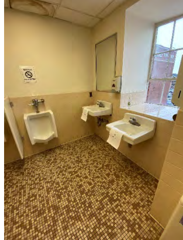
3 rd Floor Men's Toilet Room Sinks
