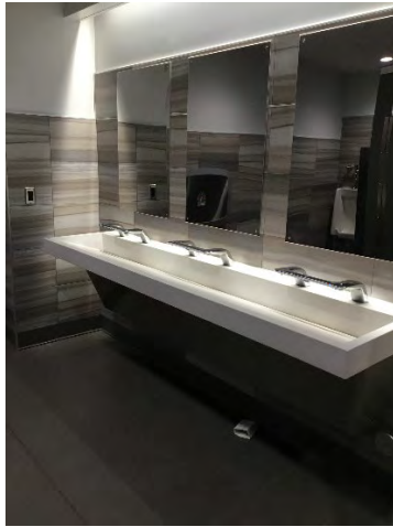
Men's Toilet Room Sinks
