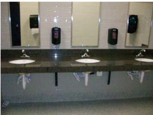
Women's Locker Room Sinks
