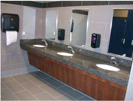
Women's Toilet Room Sinks
