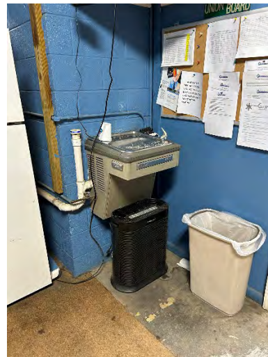
Drinking Fountain (Not in Operation)
