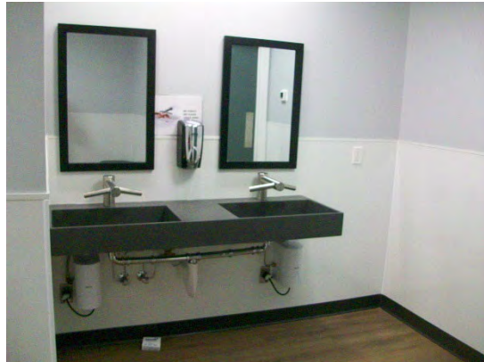
Women's Toilet Room Sinks
