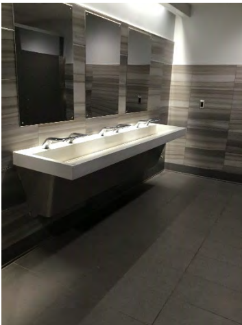
Women's Toilet Room Sinks
