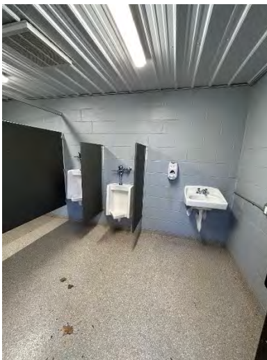
Men's Toilet Room Sink
