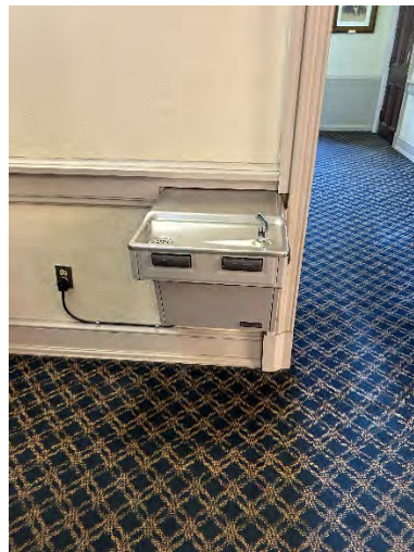
2 nd Floor Drinking Fountain
