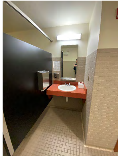
Women's Toilet Room Sink
