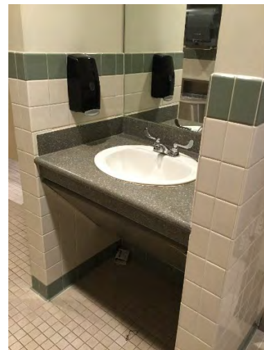
Men's Toilet Room Sink
