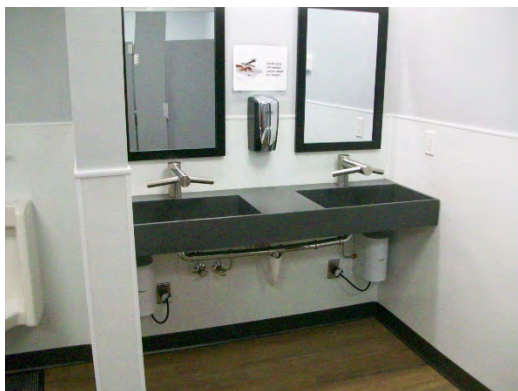
Men's Toilet Room Sinks
