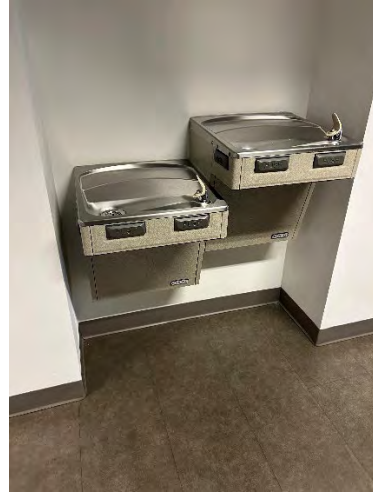
2 nd Floor Drinking Fountains
