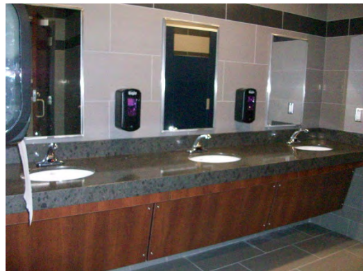
Men's Toilet Room Sinks
