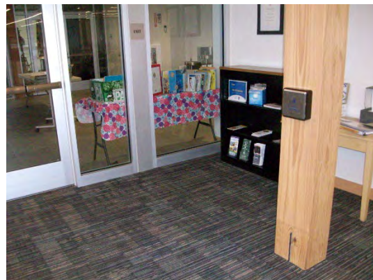
Interior Entrance Automatic Door Control
