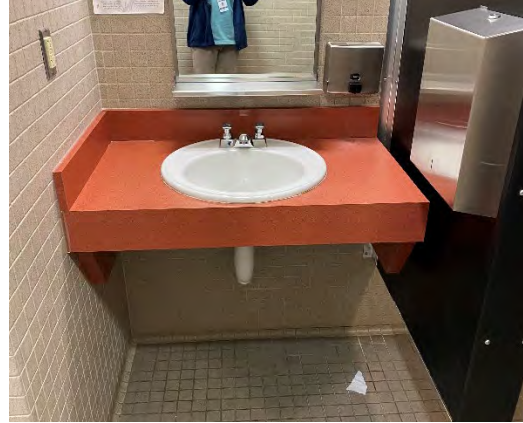
Men's Toilet Room Sink
