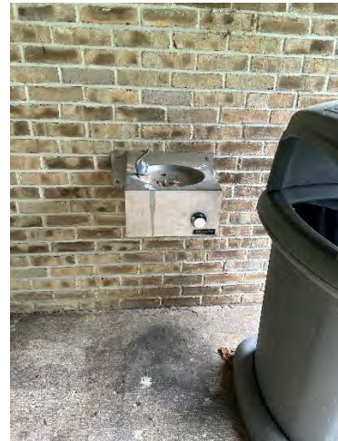
Drinking Fountain (Not in Operation)
