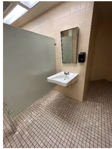
Women's Toilet Room Sink
