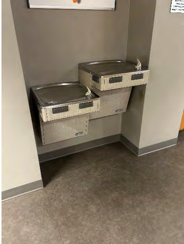
1 st Floor Drinking Fountains
