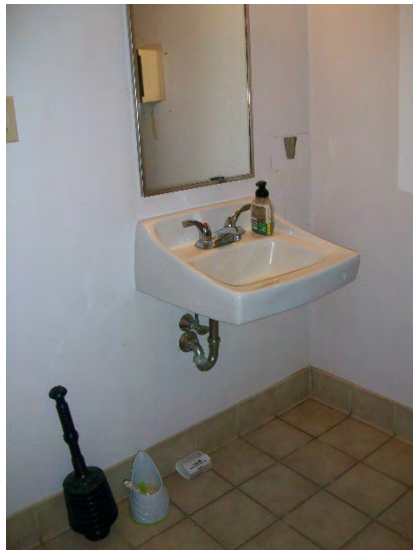
Men's Toilet Room Sink
