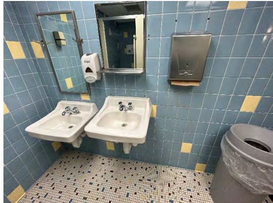
3 rd Floor Women's Toilet Room Sinks
