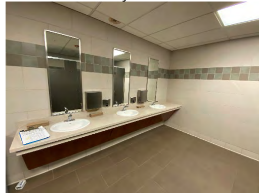
1 st Floor Women's Toilet Room Sinks
