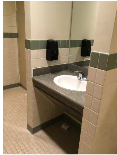
Women's Toilet Room Sink
