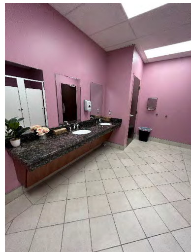
Front Women's Toilet Room Sinks
