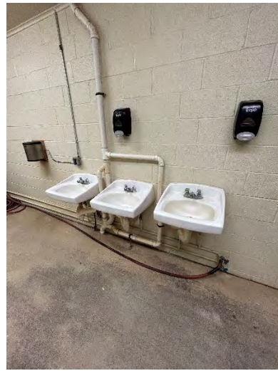
Men's Toilet Room Sinks
